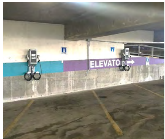
Figure 25: Low-cost wall mounted EVSE in mall parking garage
