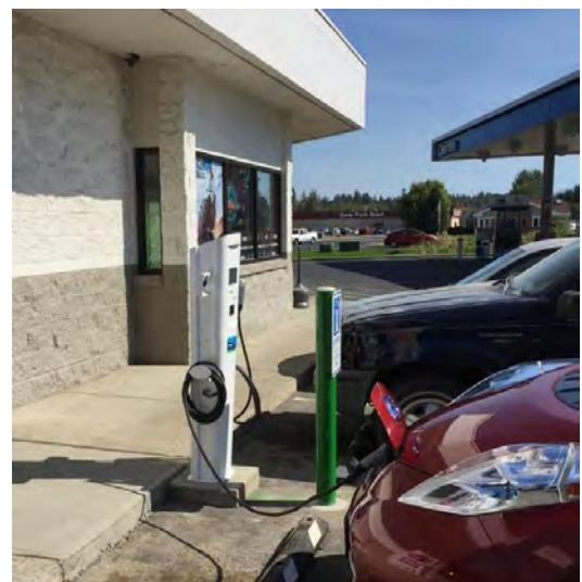
Figure 24: Public EVSE installation
