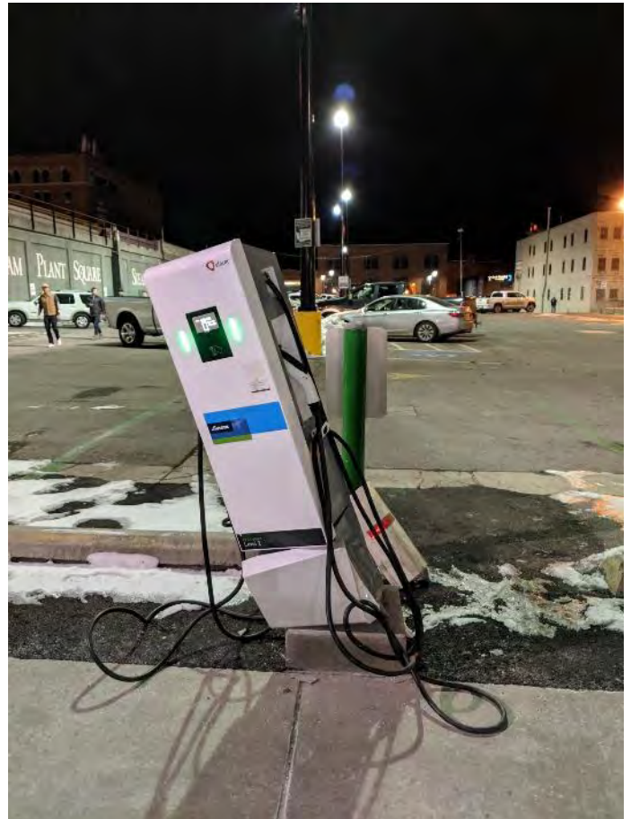
Figure 31. EVSE damage from a vehicle impact
